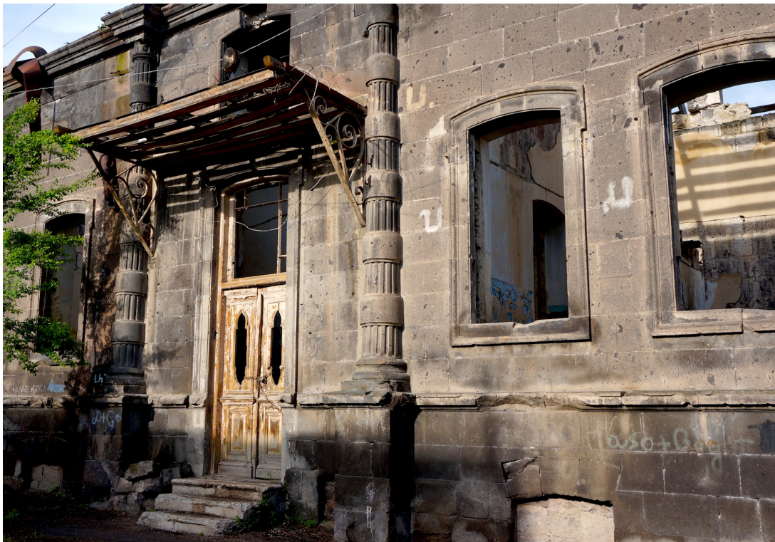
Damaged historic residence in Gyumri's Kumayri historic district.
